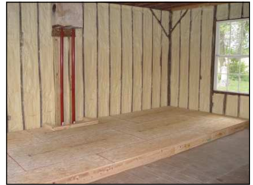
Foam insulation now protects the walls, and the chancel is ready for carpet.
