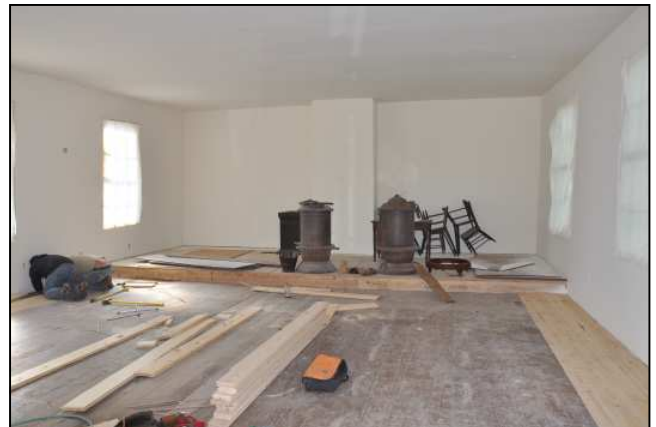
Workers finish restoring and strengthening the wood flooring on the 158-year-old structure.
